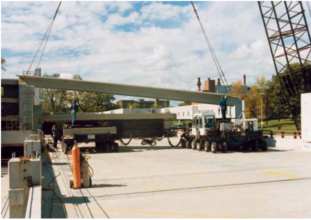
Figure 1.2.25 Special erection equipment is available for adding floors to existing parking structures.
