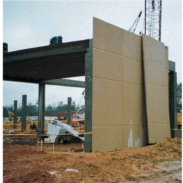
Figure 1.2.12 Erection of precast concrete wall panels is fast and can be performed year round even in cold climates. Roof diaphragms and supporting beams and columns are often also precast concrete.
