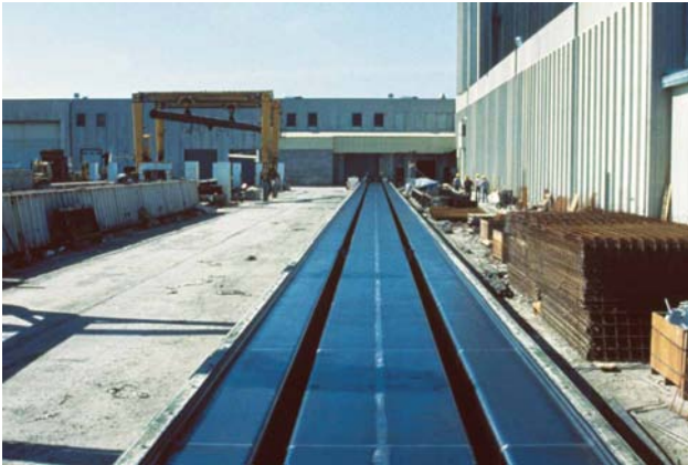
Figure 1.1.2 Long-line prestressed double tee casting bed.
