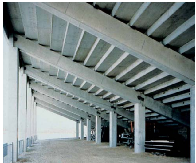
Figure 1.2.39 Repetition, simplicity and multiple form use allow the columns, raker beams and riser units to be framed economically with total precast concrete.
