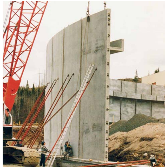
Figure 1.2.51 This large circular storage tank is under construction. Vertically prestressed precast concrete wall segments are braced temporarily. Cast-in-place concrete joints and circumferential post-tensioning complete the structure.
